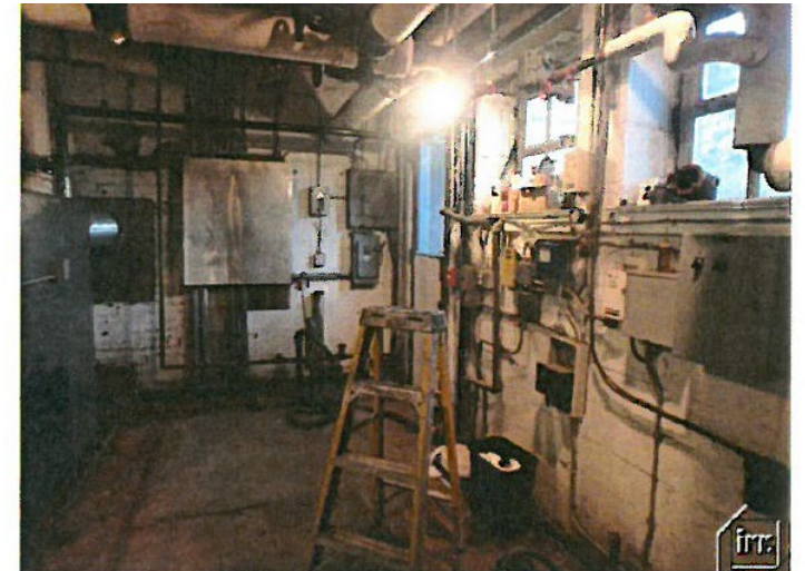
Building systems room on lower level (Photo Taken on December 4, 2018)
